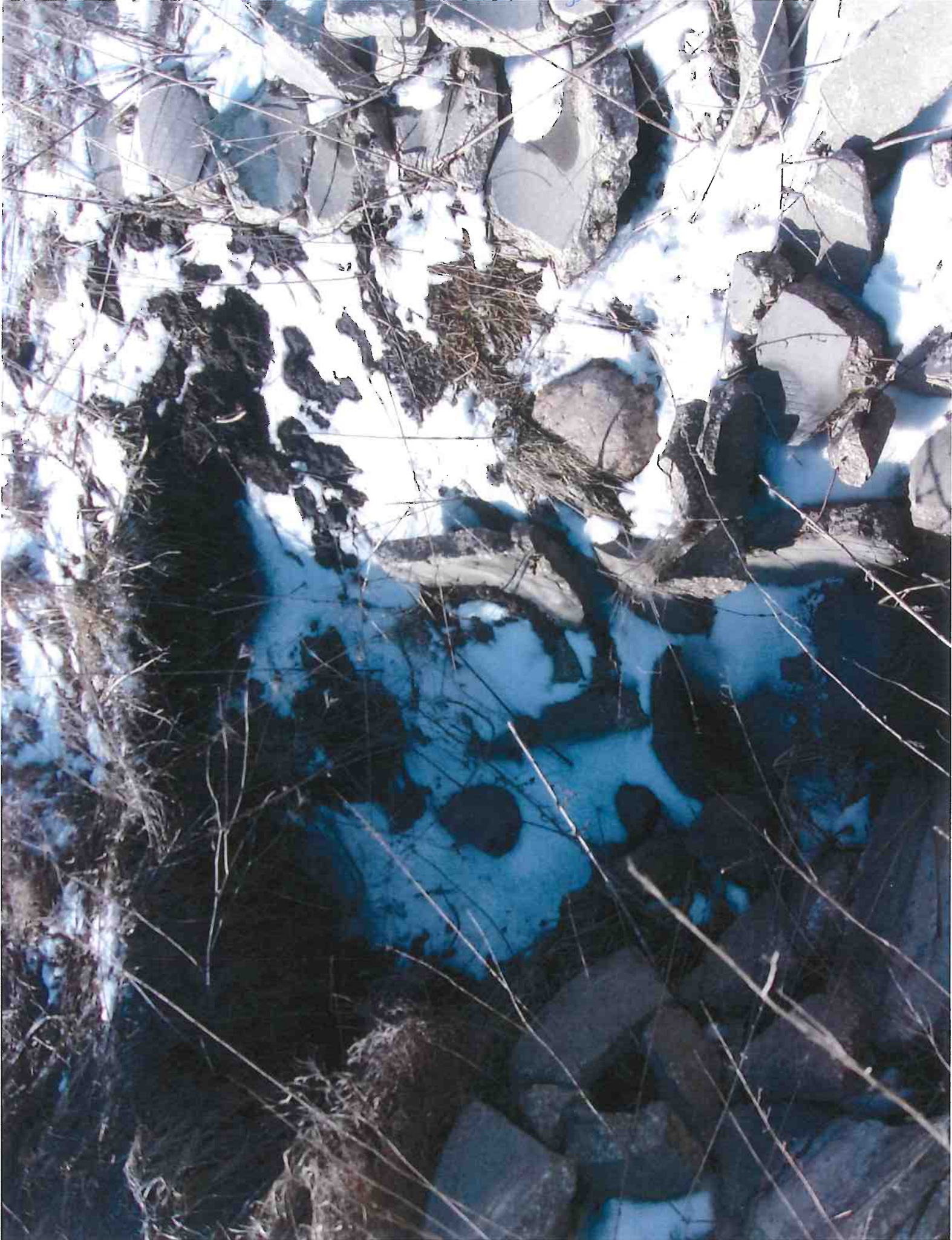
TILE COLLAPSED @ N SIDE OF D65 OLD CLAY/CMO OUTLET
